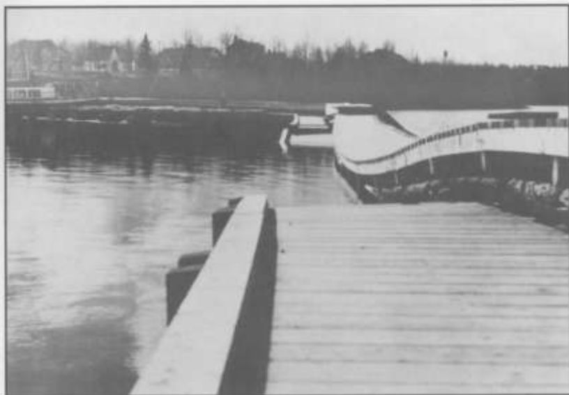
Repairs and improvements to the breakwater had no sooner been completed when it was damaged by a severe wind storm in October 1935 (credit: NAC PA119642)
